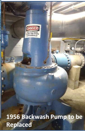
1956 Backwash Pump Motor
