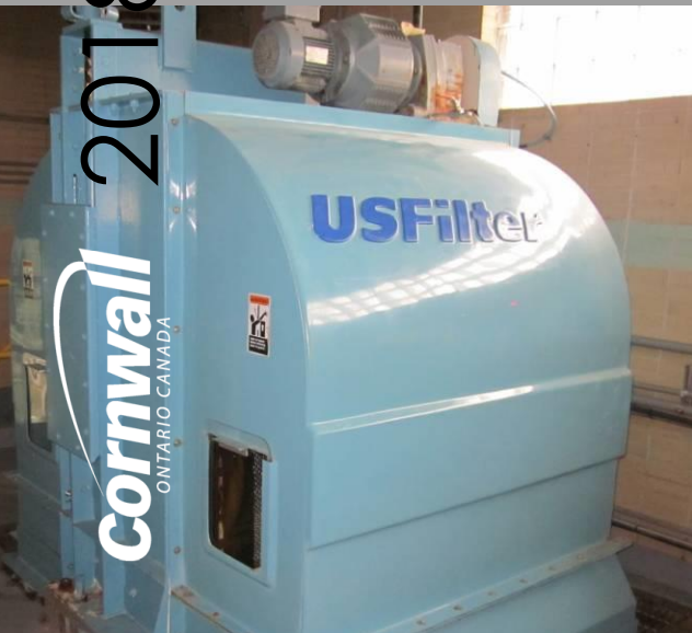
Water Purification Plant, Motorized Traveling Screen, 2011
