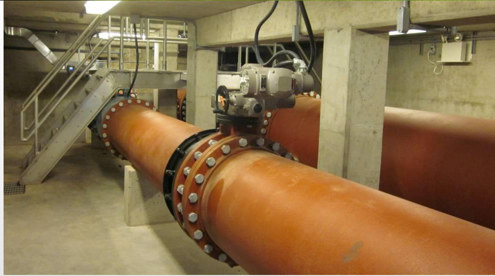
Water Purification Plant, Flow Control Chamber, 2011
