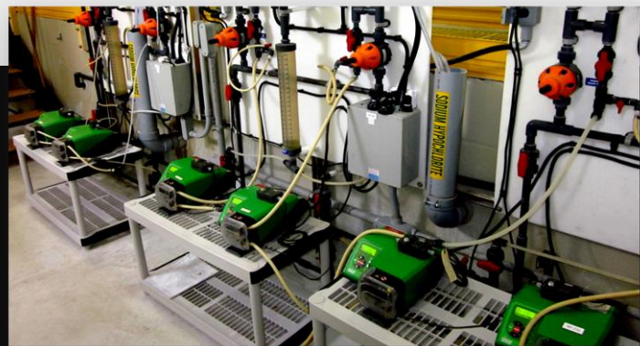
Water Purification Plant, Sodium Hypochlorite Injection System, 2018
