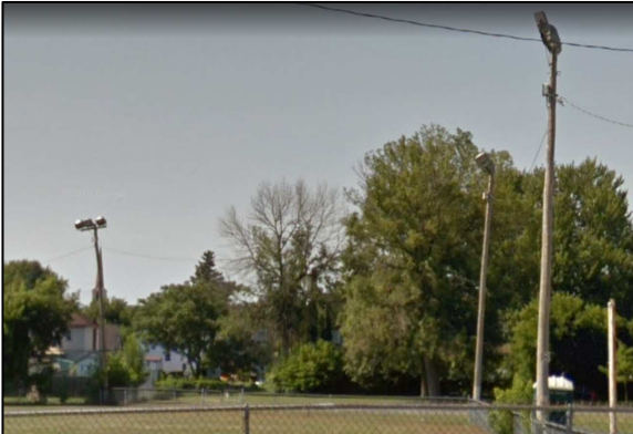
Existing wooden poles in the outfield which are no longer plumb
