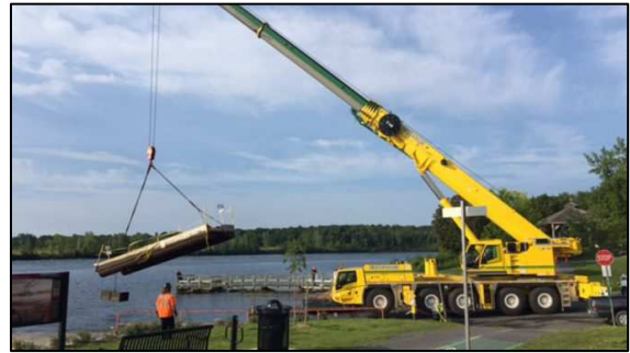
A dock at RCAF being removed by crane for the purposes of a repair in August 2017.
