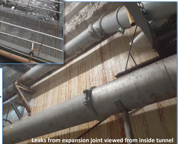
Leaks from expansion joint viewed from inside tunnel
