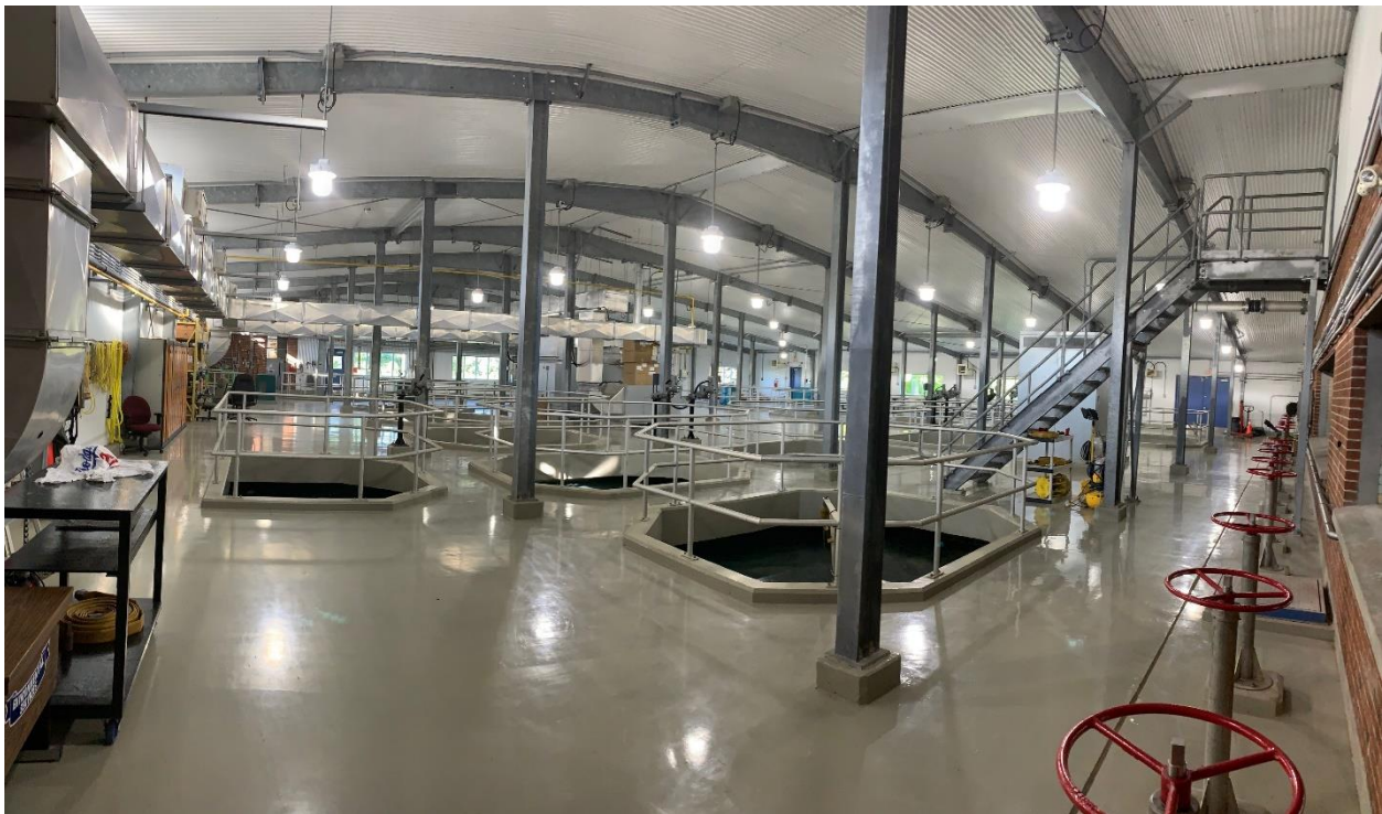
Figure 5: New and efficient LED lights installed at Water Purification Plant (WPP)
