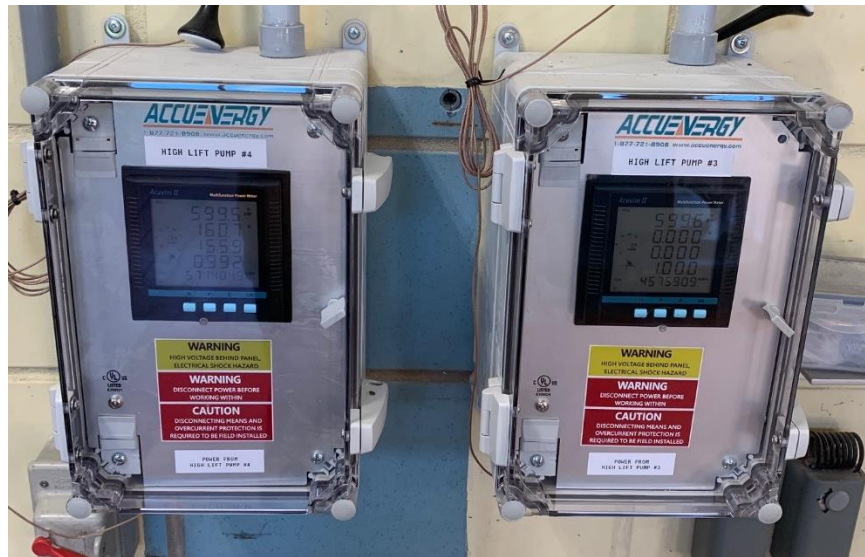
Figure 4: Smart meters installed at Water Purification Plant (WPP) for tracking real time energy consumption
